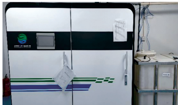
3D Medicines Beijing Laboratory sewage treatment device 思路迪北京實驗室污水處理裝置
